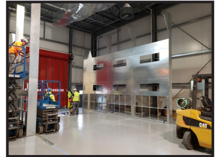
The new paint mixing booth is in the process of being installed.
